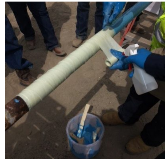
ClockSpring|NRI trained and certified technician apply Contour WA™ to a prepared line.
