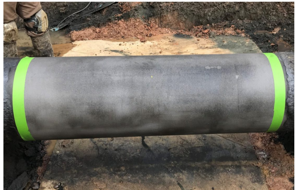
Technicians grit blasted the damaged area of the pipe and wiped it with acetone to prepare the surface for composite installation.
